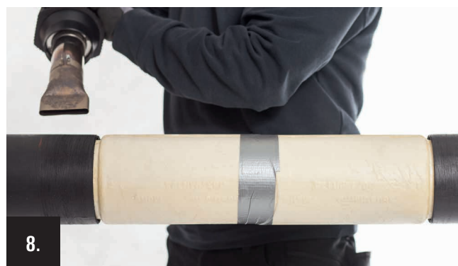
8. Attaching the shrink film: Heat cleaned casing pipe ends (with a soft flame when using a propane gas burner) to approx. 80 ° C. Check the temperature before installing the shrink film.
