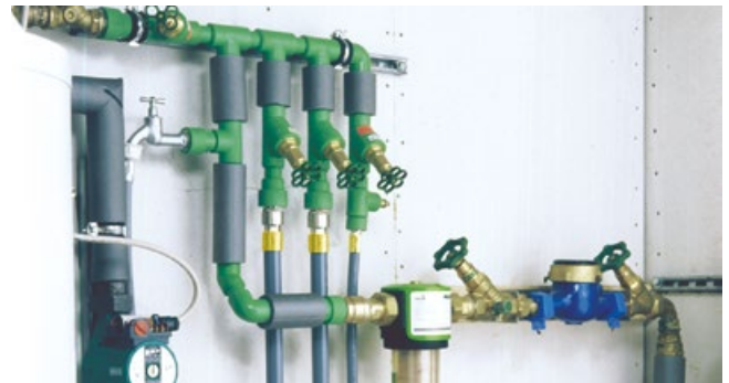
House connection station
