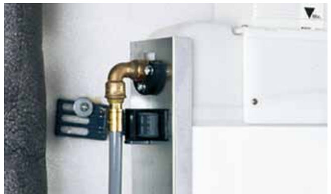
Potable water installation
